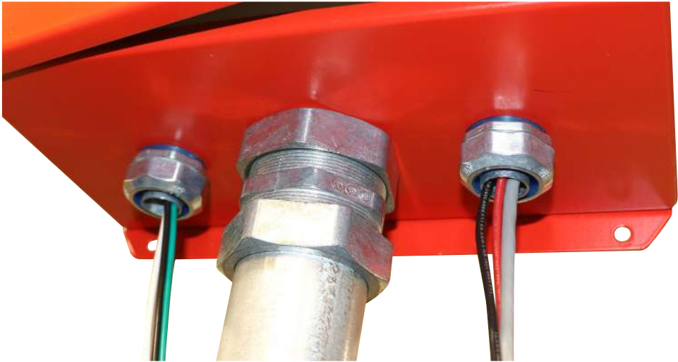
AC Connection Wires From PCU
